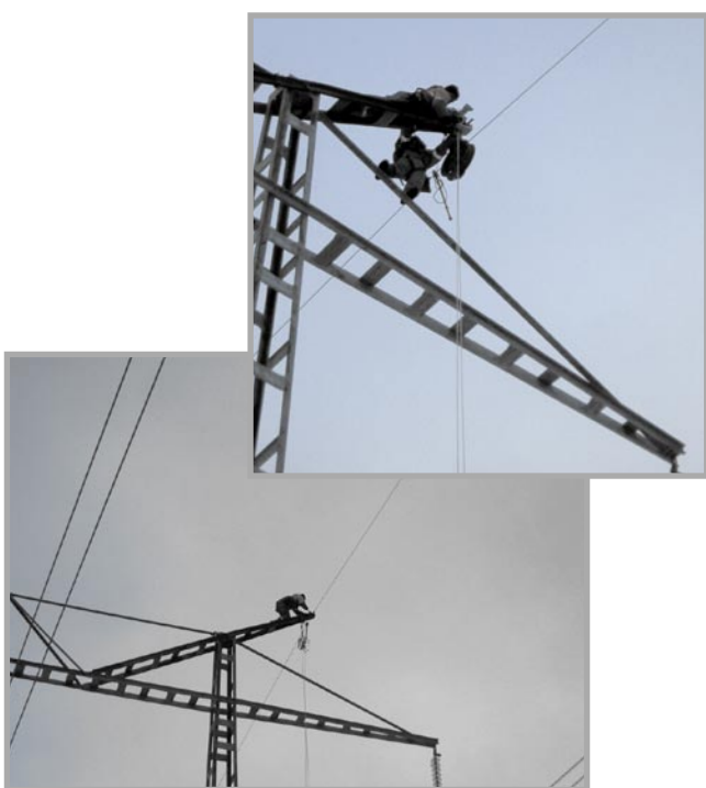
Fig. 6. Placing earthing conductor on pulley-blocks on active 400 kV power line (Polish work team task performed in the Sweden)
