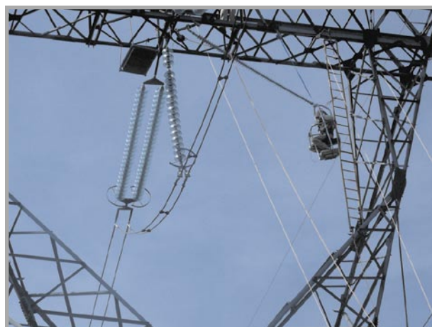
Fig. 4. Preparing presentation for ICOLIM 2008 – insulator chain exchange with use of by composite insulator suspended cabin
