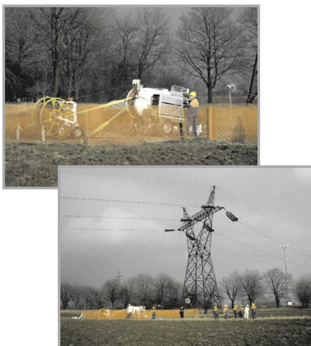
Fig. 7. Preparation for earthing conductor exchange to OPGW (training near to the Tarnów)
