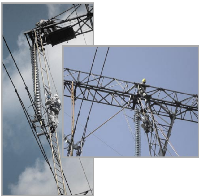
Fig. 2. Live work on insulators exchange on the 400 kV power line during the training
